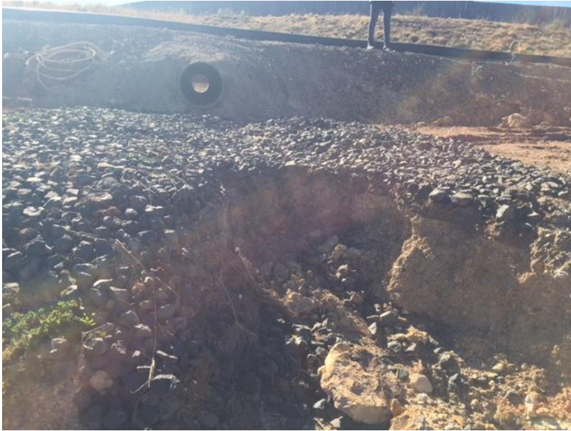
Photo 13 Additional erosion and sediment control required at culvert into Western Holding Dam
