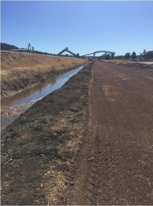
Photo 1 Window needs reshaping in areas along main access road east of Eastern Holding Dam
