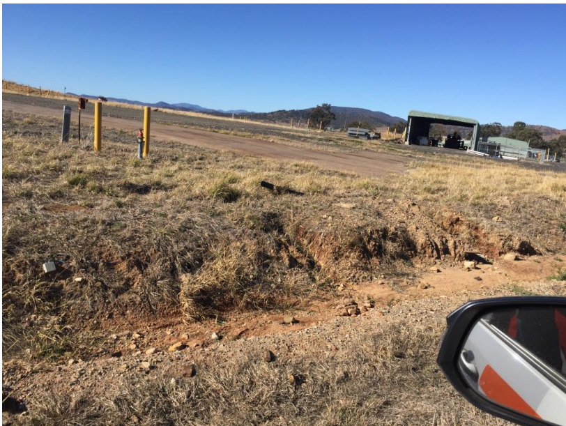
Photo 10 A section of the drainage line on the pit top main road has washed out
