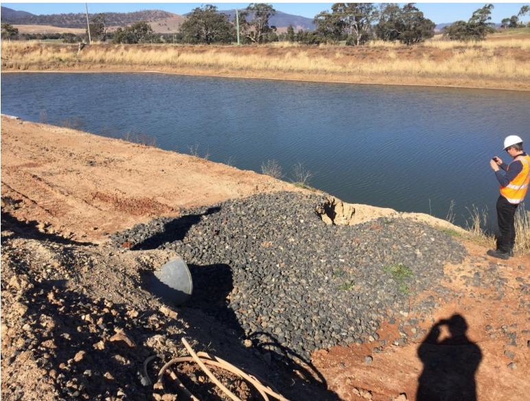
Photo 12 Additional erosion and sediment control required at culvert into Western Holding Dam
