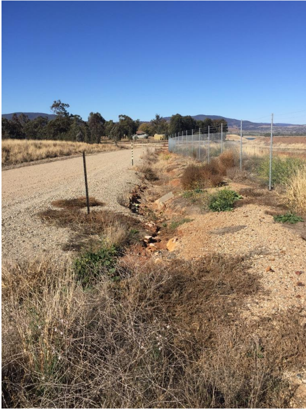
Photo 9 Drainage Line along pit top access road is not stable and needs additional erosion and sediment control design and implementation
