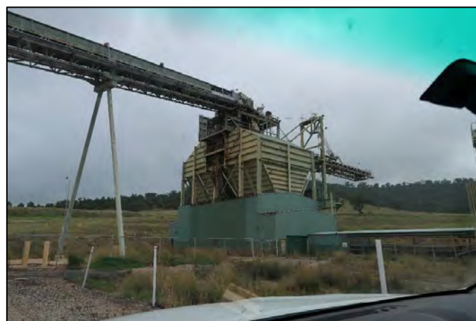
Figure 23 – Raw Coal Distribution System
